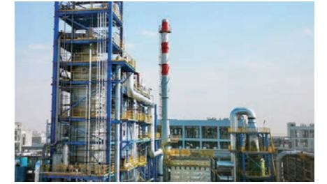
山东某精细化工行业废气液焚烧项目 Waste Liquid and Waste Gas Incineration, Fine Chemicals Industry, Shandong
