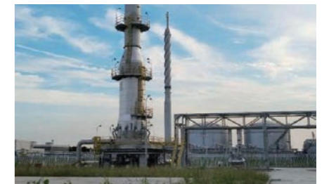
南京某罐区热氧化炉 Tank Farm Thermal Oxidizer, Nanjing
