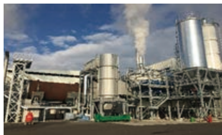
法国某危废处置装置 Hazardous Waste Treatment Facility in France
