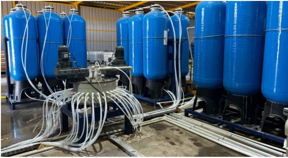
Figure 1: Pilot Plant Multi-Valve Feeding Brine to DLE Columns (approx. 2.5 metres high)
