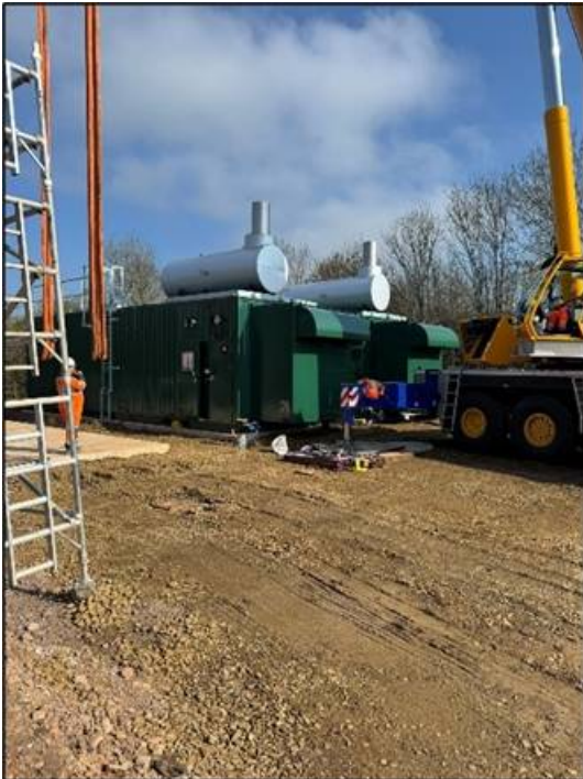
2. Rolls-Royce MTU containerised gensets installed and positioned on concrete bases on site
