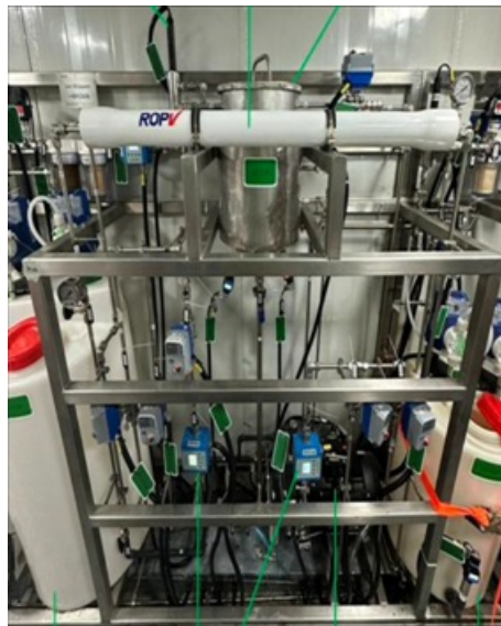
Fig. 4: Low Pressure and Medium Pressure R/O Unit (Lanshen)
