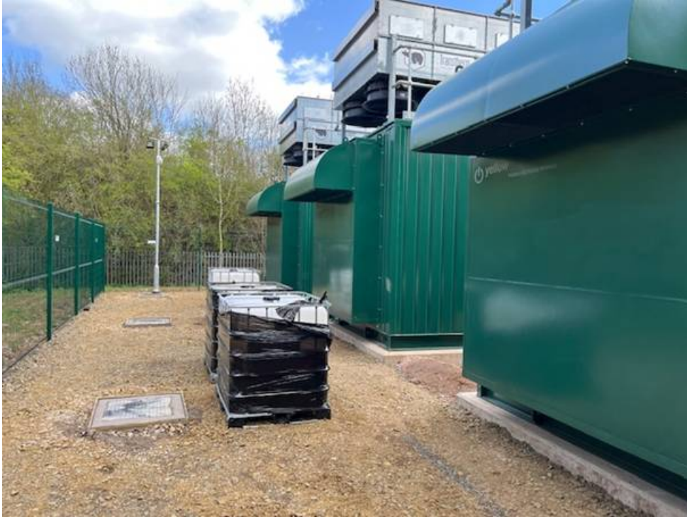
1. Completed gensets and radiator cooling packages installed on site
