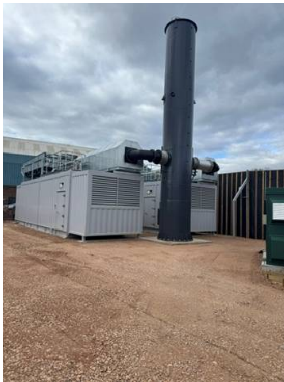
1. The two Caterpillar G3520K genset enclosures and exhaust stack
