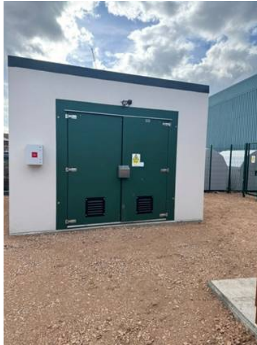
4. The completed HV switchroom
