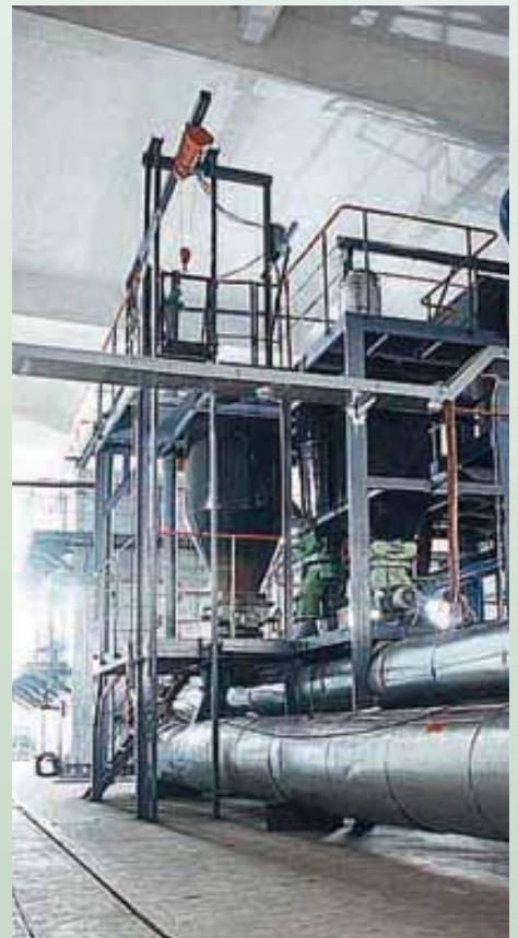
The furnace on trial operation 鍋爐實驗
