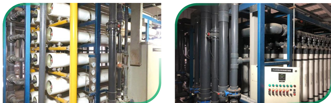
UF+ primary reverse osmosis unit
