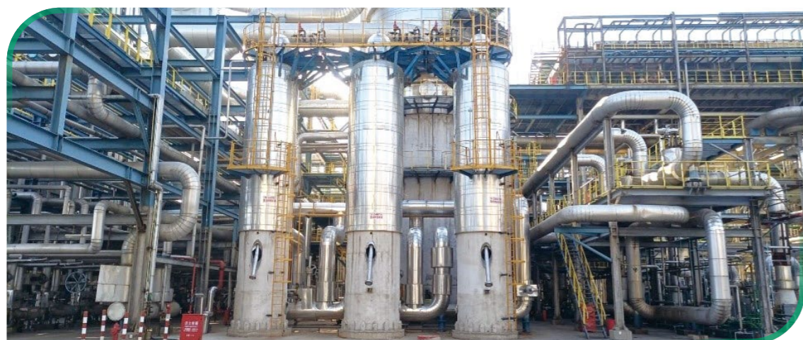
high-efficiency ultra-clean aromatics heating furnace
