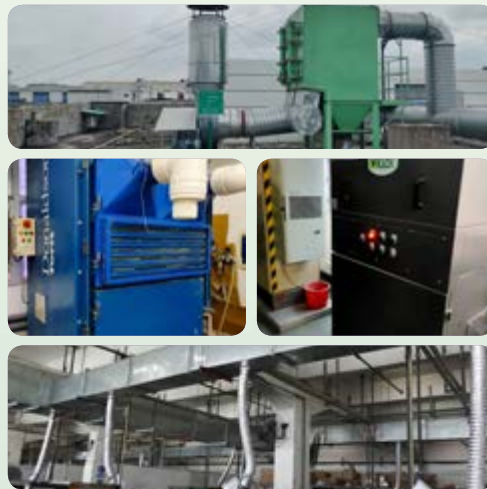
Exhaust air treatment facilities 廢氣處理設施
