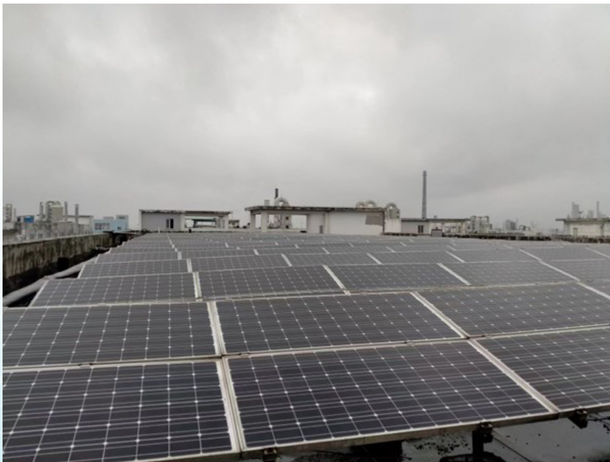
Figure 1 Solar panels installed on-site at the Eco-Plating Specialised Zone
