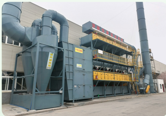
Organic waste gas catalytic combustion equipment.
