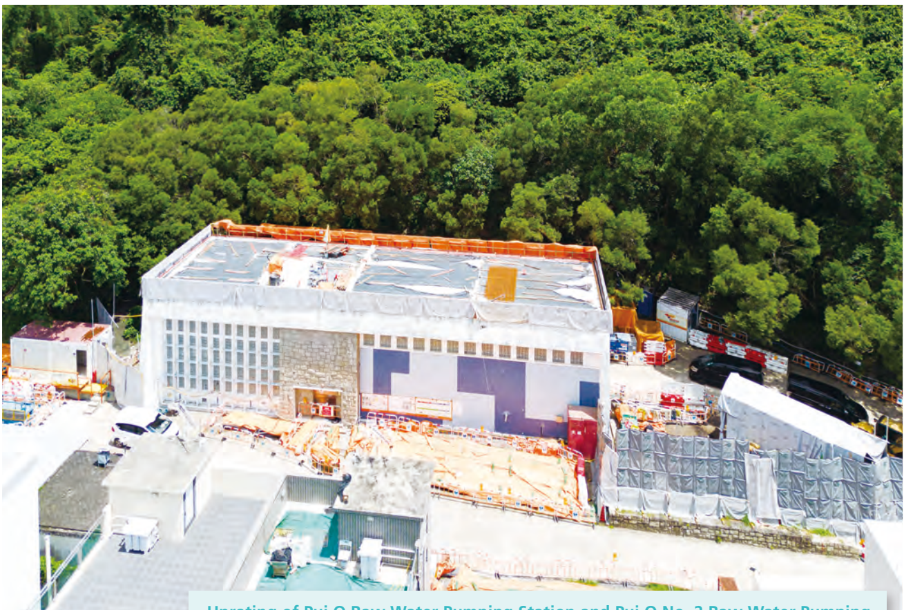
Upgrading of Pui O Raw Water Pumping Station and Pui O No. 2 Raw Water Pumping Station and Laying of Raw Water Mains along South Lantau Road 提升貝澳原水抽水站及貝澳二號原水抽水站及沿嶼南道敷設原水水管
