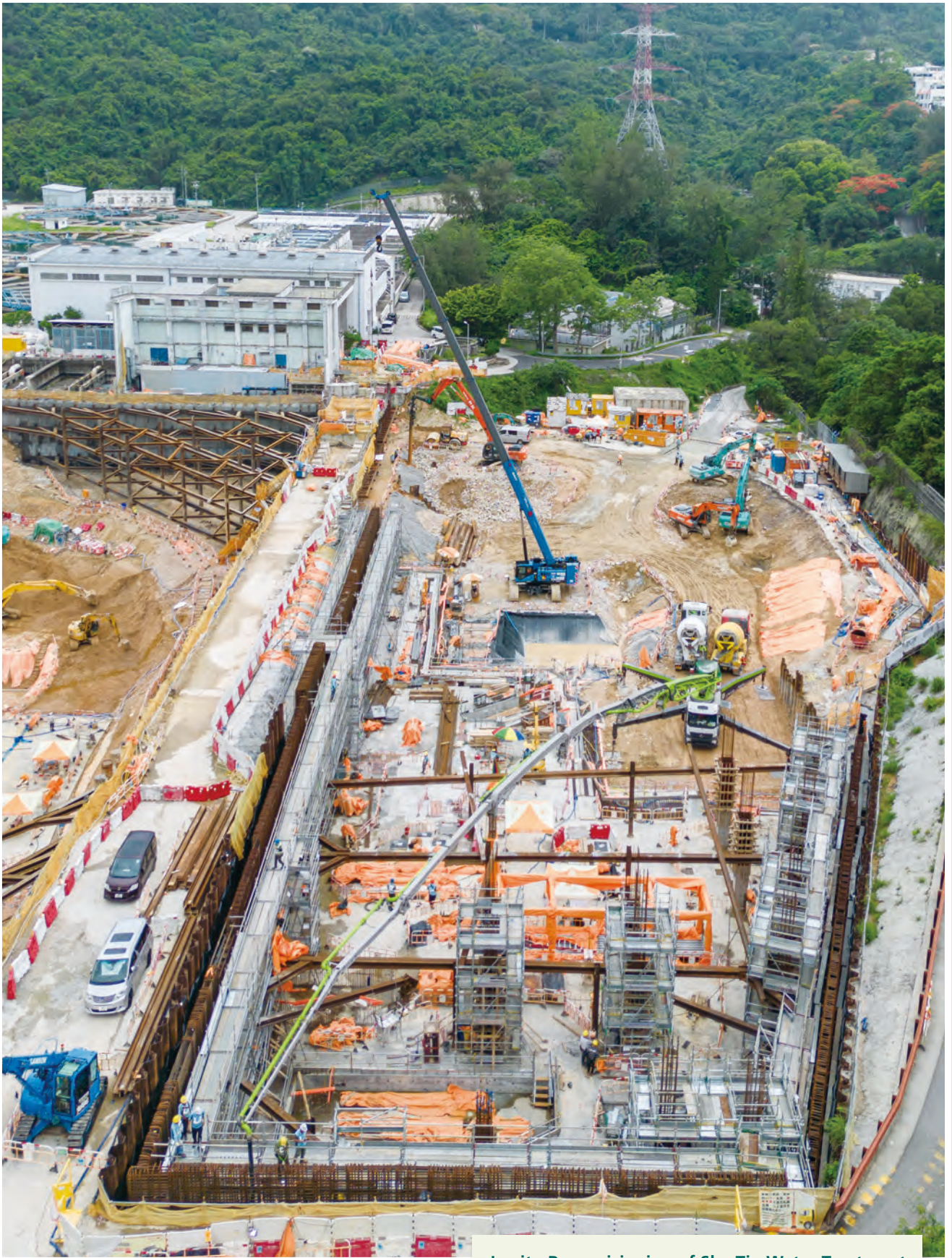
In-situ Repositioning of Sha Tin Water Treatment Works (South Works) – Administration Building 沙田濾水廠原地重置工程（南廠）－行政大樓
