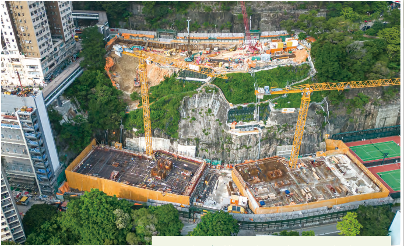
Construction of Public Housing Development at Hiu Ming Street 曉明街公營房屋發展之建造工程
