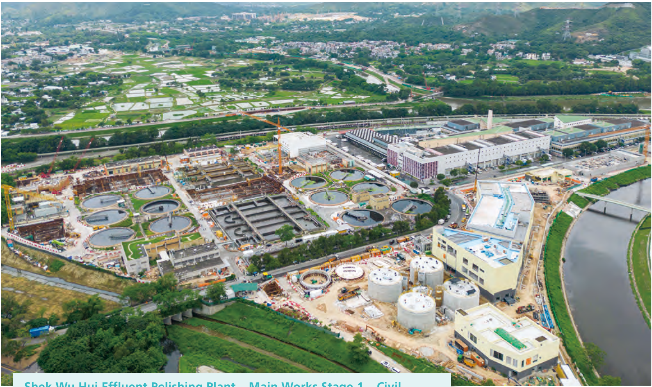
Shek Wu Hui Effluent Polishing Plant – Main Works Stage 1 – Civil Works for Sludge Treatment Facilities and 132kV Primary Substation and Civil Works for Sewage Treatment Facilities 石湖墟淨水設施－主體工程第一階段－污泥處理設施及132kV主變電站的土木工程及污水處理設施的土木工程
