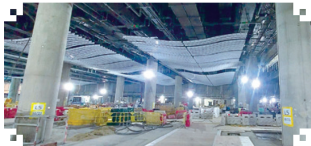
HKIA Contract 3508 Terminal 2 expansion works – Design, supply and installation of lower-level baffle and external ceiling system 香港國際機場合約3508二號客運大樓擴建工程－設計、供應及安裝低層天幕及室外天花系統
