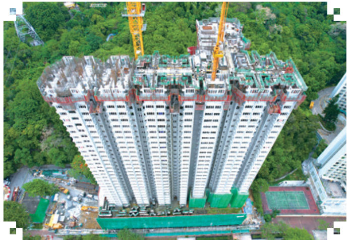
Public housing development at Hin Fat Lane, Tuen Mun 屯門顯發里之公共房屋發展項目
