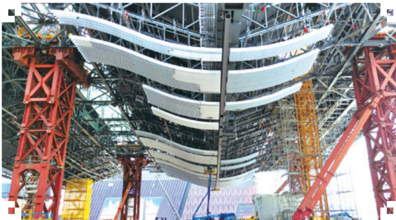
HKIA Contract 3508 Terminal 2 expansion works – Design, supply and installation of main roof baffle ceiling system 香港國際機場合約3508二號客運大樓擴建工程－設計、供應及安裝主天幕金屬天花系統
