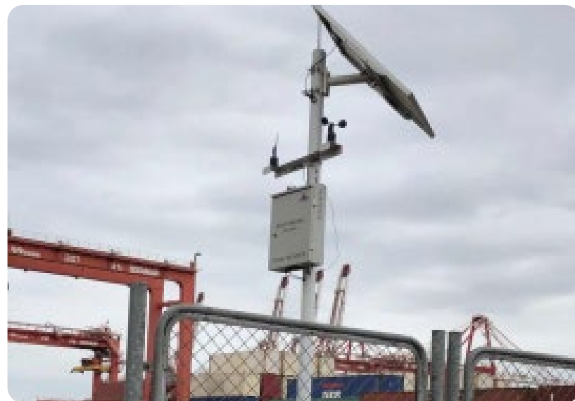
↑ Photo of Intelligent Monitoring and Control System for Ecological Environment (Atmosphere)
