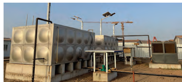
Solar Water Heating System of CBMI's SC3 Project in Senegal
