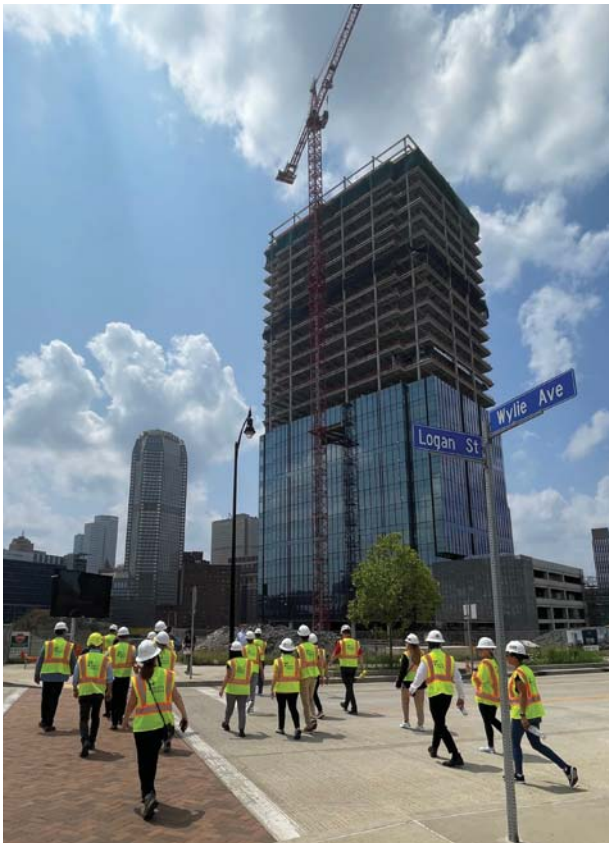
A group of FNB employees head to the FNB Financial Center site for a tour during construction.
