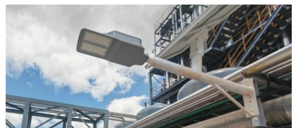
Solar PV Street Lights at Sanming Hexaflu
