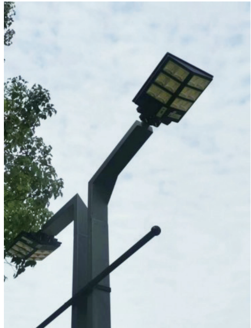
光伏路燈 Photovoltaic street lights
