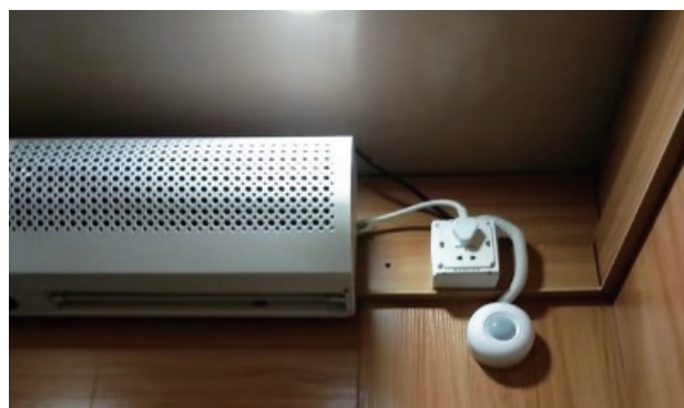
公區感應燈 Sensor lights in public area
