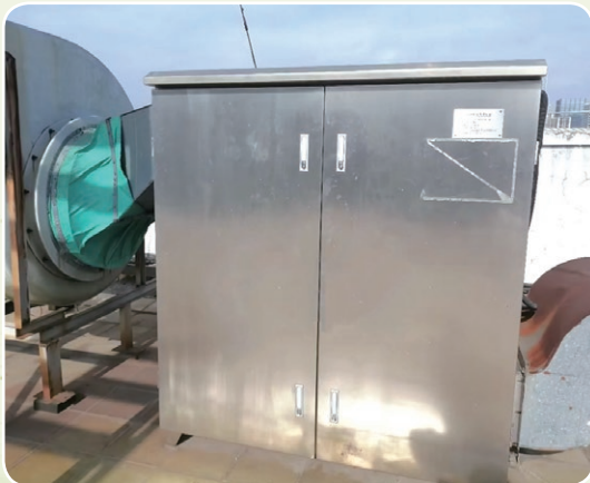
Before the renovation of the printing treatment exhaust gas system 印刷處理廢氣系統改造前
