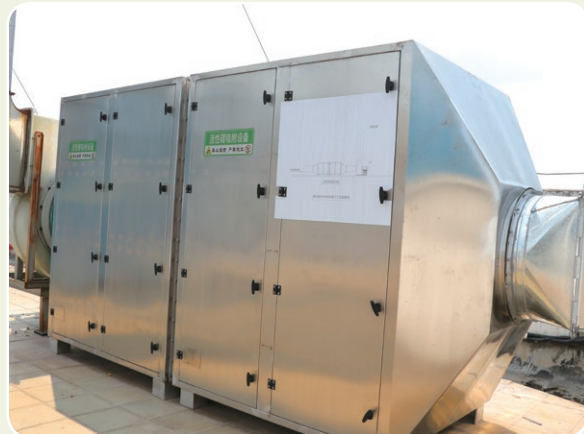
After the renovation of the printing treatment exhaust gas system 印刷處理廢氣系統改造後
