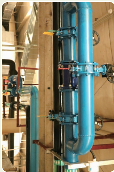
Renovation of the cooling water tower in Building G G棟冷卻水塔改造
