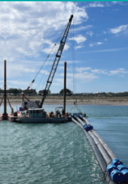
Investment in new deeper intake piping to improve resiliency for the Park Shores Water Treatment Facility in Comal County, Texas
