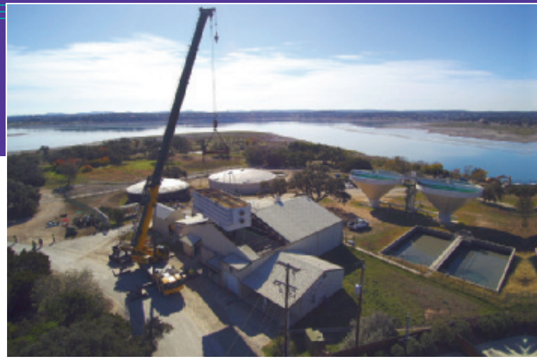
Investing in a filter replacement in Comal County, Texas
