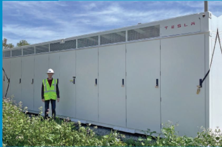
BESS on-site at San Jose Water Company's Williams Station
