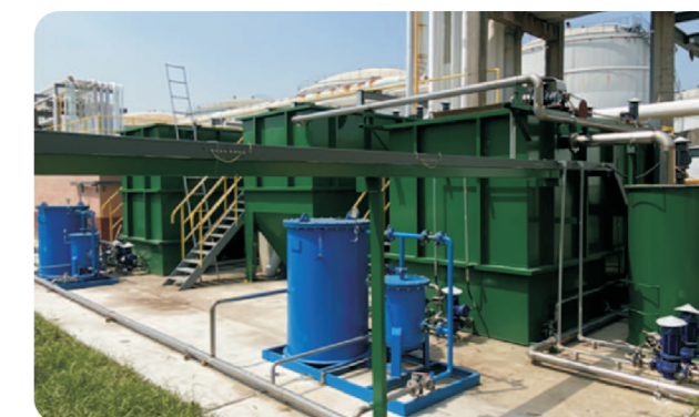
Taicang Power Shell Petrochemical Co., Ltd. cleaning station
