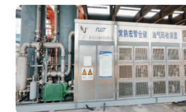
The Changshu Great Smart Petrochemical Terminal has recently procured new oil and gas recovery equipment.
