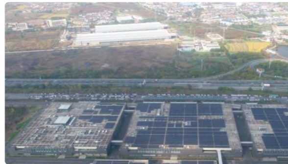
The Heyang photovoltaic project, with an installed capacity of 5.724MWp, generated 7.605 million kilowatt-hours of electricity in 2023, surpassing the annual target of 5.884 million kilowatt-hours.
