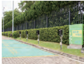
Electric vehicle charging areas 電動車充電專區
