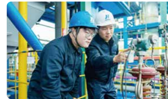
Automatic control and regulation of the entire process of sewage treatment system
