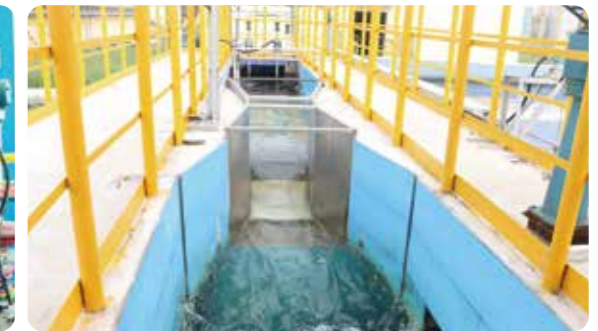
Discharge outlet of sewage treatment plant
