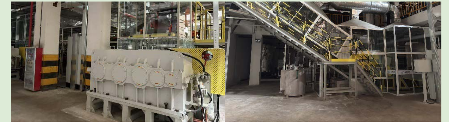
Exhaust Gas Collection Device
