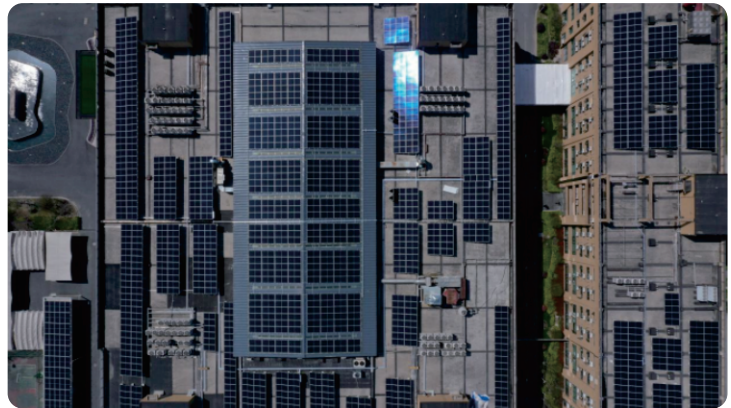
Hangzhou Photovoltaic Project
