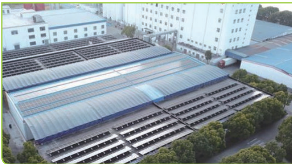
◇ The 0.7-MW solar PV modules installed in the flour mill in Jintan 於金壇麵粉廠所安裝0.7兆瓦的太陽能光伏組件
