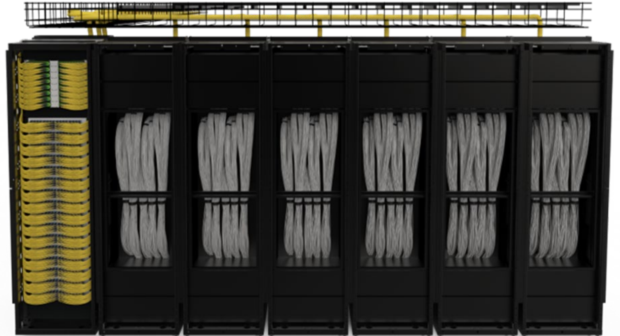
Switch Rack and Back of Six Server Racks
