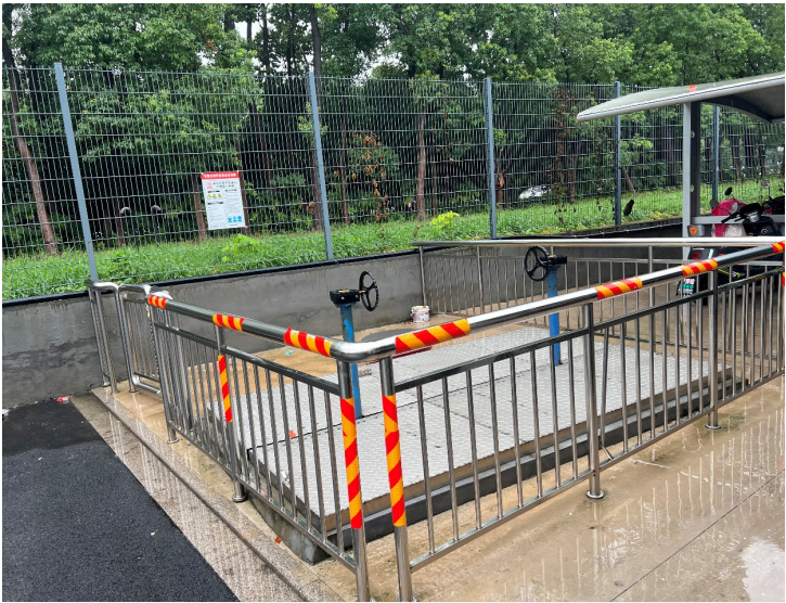
Photos of the Rainwater Pool and the Fire Water Pool
