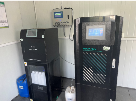
Rainwater online equipment - monitoring factor total phosphorus
