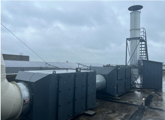
New waste gas treatment equipment Auxiliary Six (mechanical oil removal + activated carbon adsorption)
