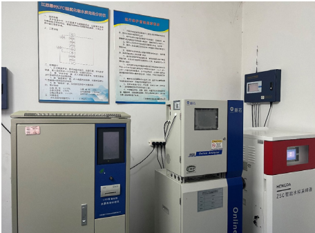
Wastewater online equipment - Monitoring factors COD, Ph, chloride
