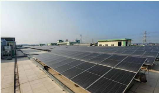
Photovoltaic Project of Guangdong Anjoy
