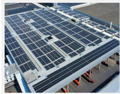
Roof Photovoltaic of Nine Tech Co., Ltd.
