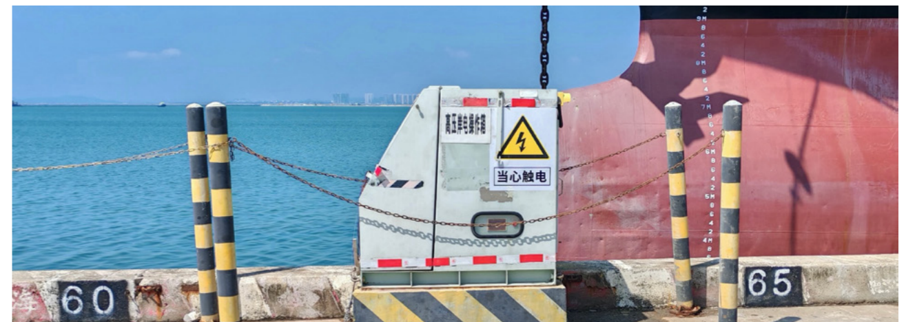
Shantou Port High-Voltage Shore Power Equipment
