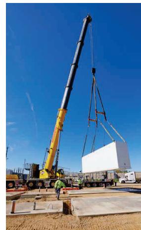
A future-forward electric grid is safe, reliable, adaptable and resilient. In the fall, MGE installed 7-MW batteries at three different locations across its distribution system. These batteries provide enhanced reliability and stability on our community grid from various points on the system.
