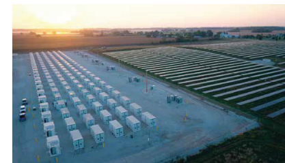
In June, Wisconsin's first large-scale battery energy storage project came online. MGE owns 10% of the 200-MW solar array and the 110-MW battery storage system at the Paris Solar-Battery Park in Kenosha County. The batteries store renewable energy that can be dispatched when needed to maintain grid stability.
