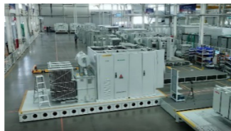
Workshop Finished Products Transfer
