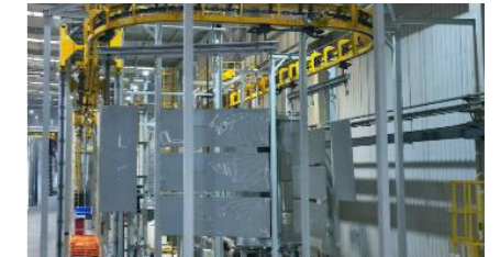
Waste Heat Recovery System
