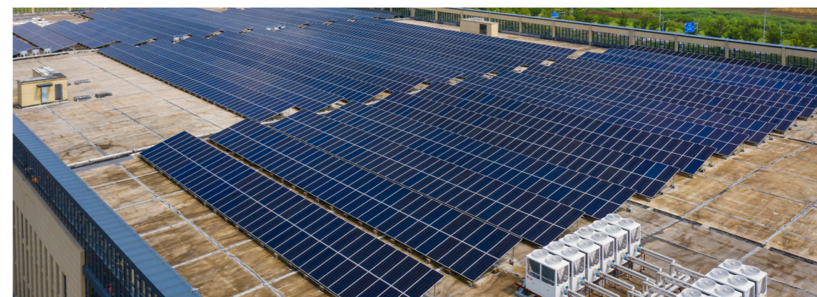
▲ Rooftop Photovoltaic Project of Ningxia JingHuan
