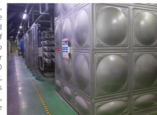
▲ Reclaimed Water Station
