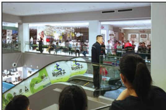
Escalator emergency response training at Mianyang Fulin Parkson 綿陽富臨百盛手扶電梯應急處理培訓
