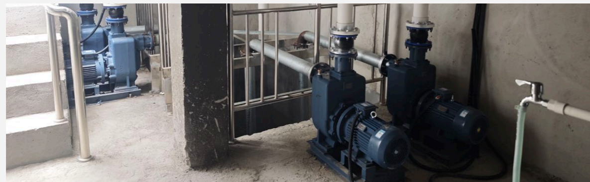
Closed-Loop Wastewater Recycling System for Coating Lines
