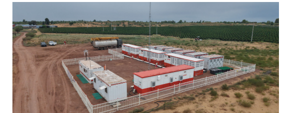
"Small Grid + Storage" Solution in Jereh Agile Power Energy
