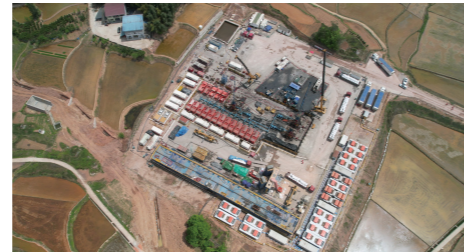
Operation Site of AI•R FRAC Intelligent Fracturing System
