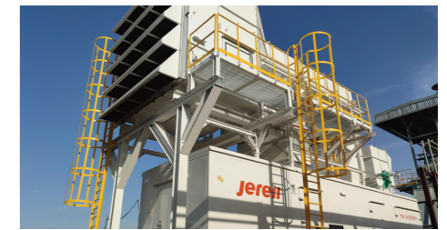
Gas Turbine Hydrogen-Doped Combustion for Power Generation
