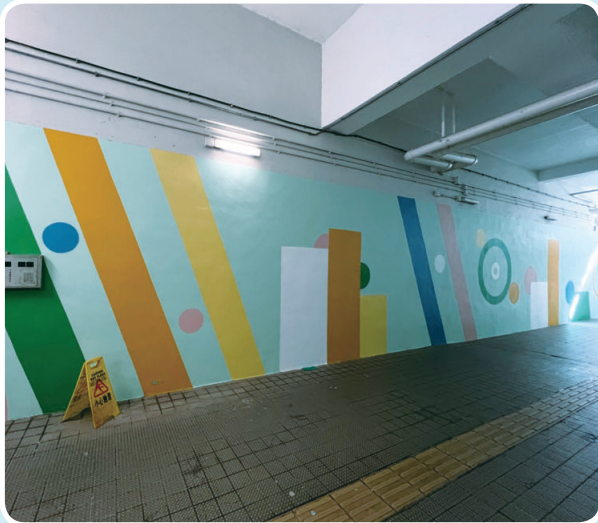
Description: Well-being Improvement Works at Kwai Shue House in Lei Muk Shue (II) Estate
