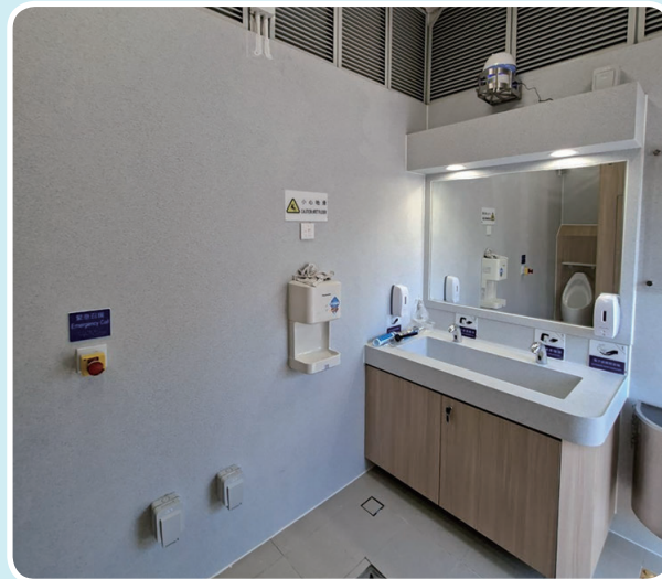
Description: Replacement of counter top including basin, electronic sensor water taps and pipework 描述：更換檯面，包括洗手盆、電子感應水龍頭和管道工程
