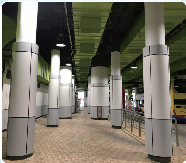
Description: Repainting of Metal Cladding Columns, at South Horizons Public Transport Interchange 描述：海怡半島公共運輸交匯處金屬柱重新噴漆
