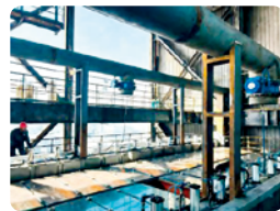
Optimization and renovation of the No.1 pulverizing system of the No.1 blast furnace
