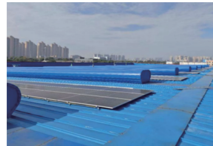
Rooftop Photovoltaic System
