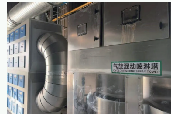
Exhaust Gas Treatment Facilities
