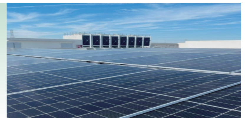
Distributed Photovoltaic System
