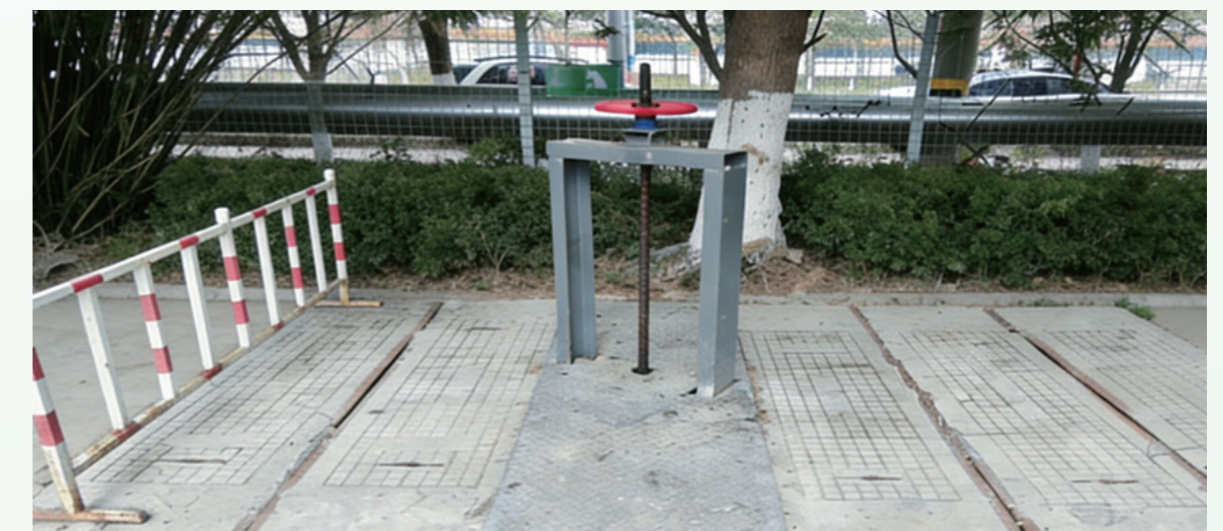
Rainwater Collection Basin on Site
