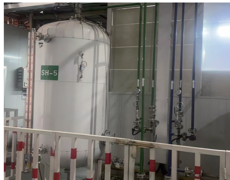
On-site Centralized Oil Supply Tank
