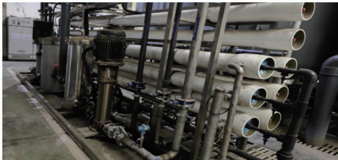
Recycled Water Reuse Membrane Modules
