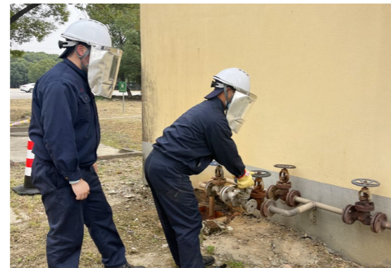
Emergency Drill for Steam Pipeline Leakage Incident
