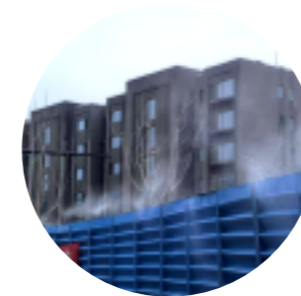
围墙及安全通道喷淋
