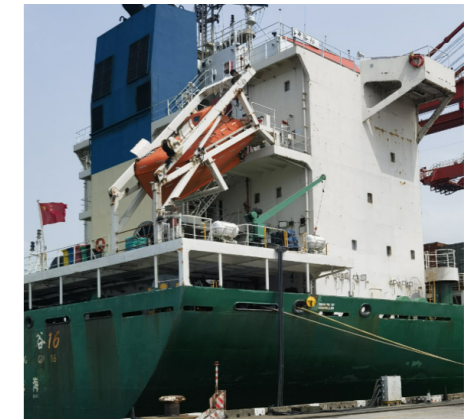
Ship Shore Power Installation
