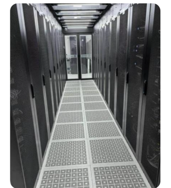
The Company's server room
