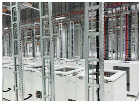
Immersion Liquid Cooling System for a Data Center in Malaysia
