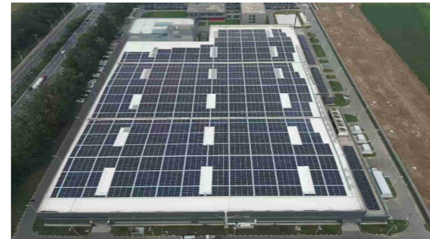
Photovoltaic Rooftop at Tianjin SofTool
