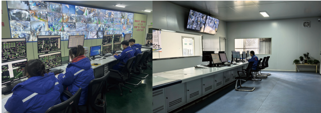
Digital and intelligent construction of Northeast Fufeng, and automatic control room of Baoji Fufeng 東北阜豐智能化數字化建設、寶雞阜豐自動化控制室
