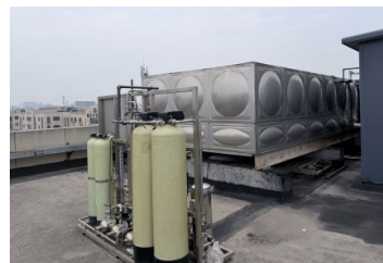
⬆️ Jiaxing Shuanghuan Wastewater Recycling Equipment
