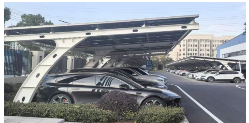
↑ Carport Rooftop Photovoltaic Photo
