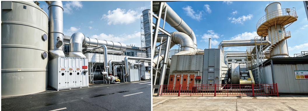
Air Pollution Treatment Equipment 廢氣處理設備
